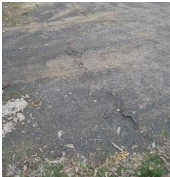
Fig. 4.14 Surface Compression Buckling Observed in a Pavement
