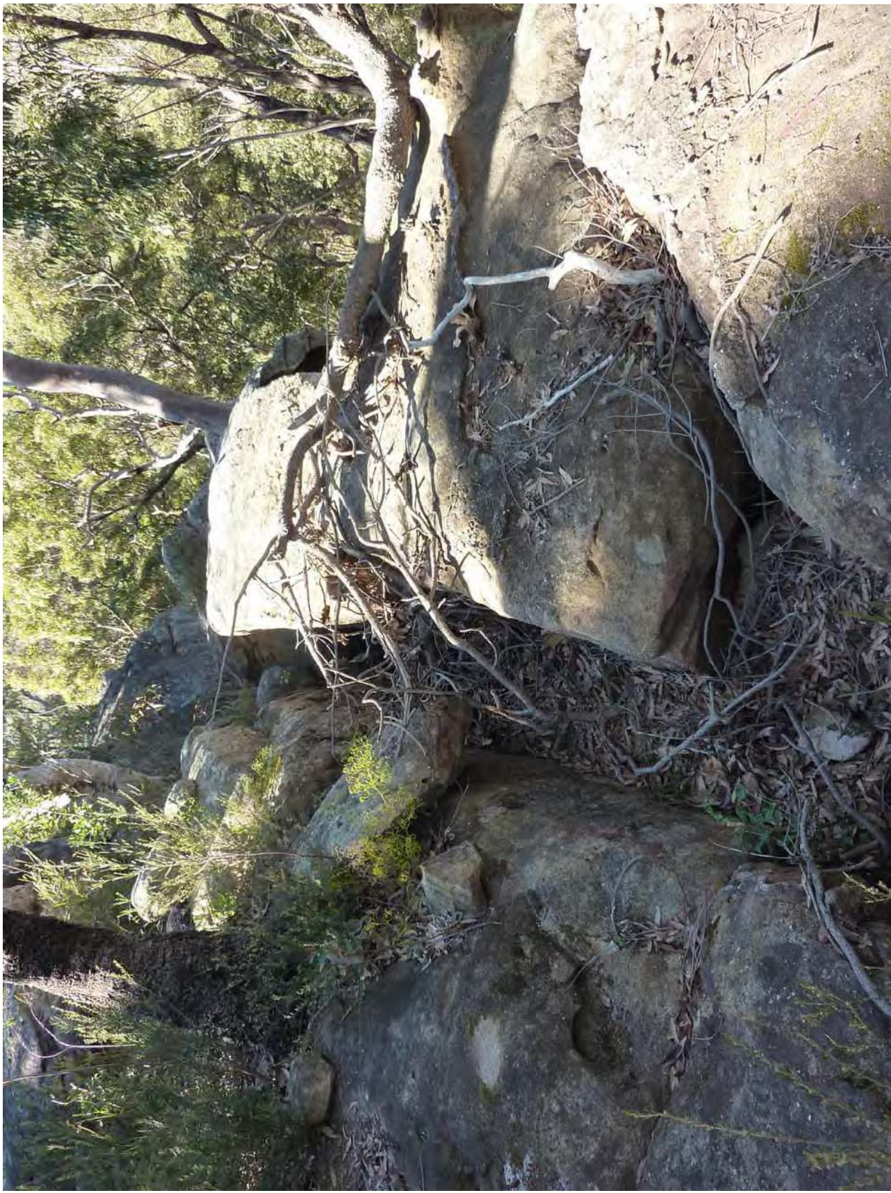
Photo C14-02 Detached blocks at western end of COH14
